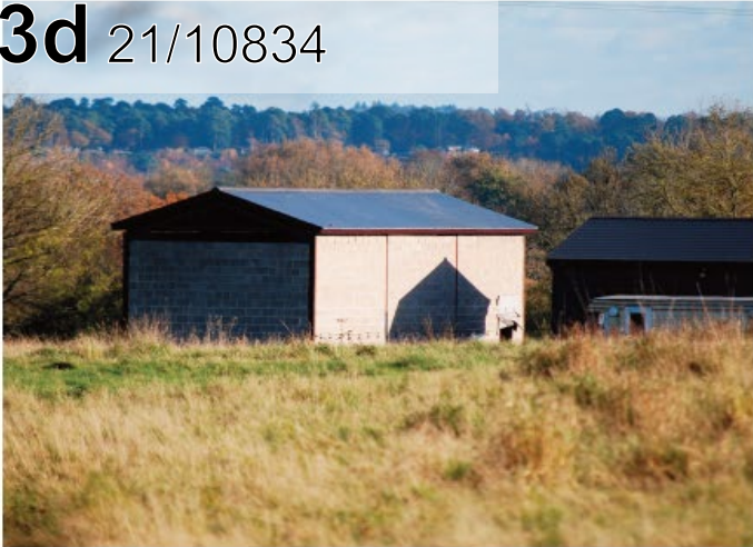
West view from woodland - illustrating Block Work to roof line, plus brand new slate roof, door entrance lower right corner
