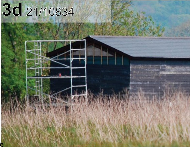
West view from woodland - illustrating continued works to insulate and clad building 24.04.2020
