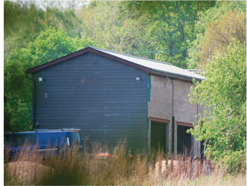
North East view from adjoining farmland (with permission) - illustrating continued works to insulate and clad building 24.04.2020
