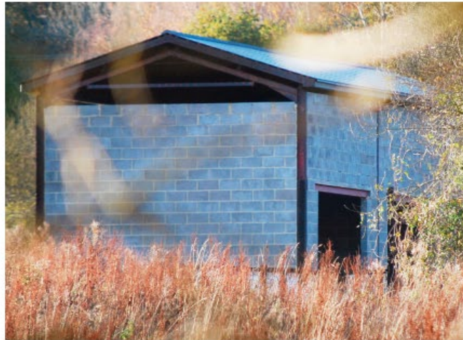
North East view from adjoining farmland (with permission) illustrating block work, plus one of three large openings.
